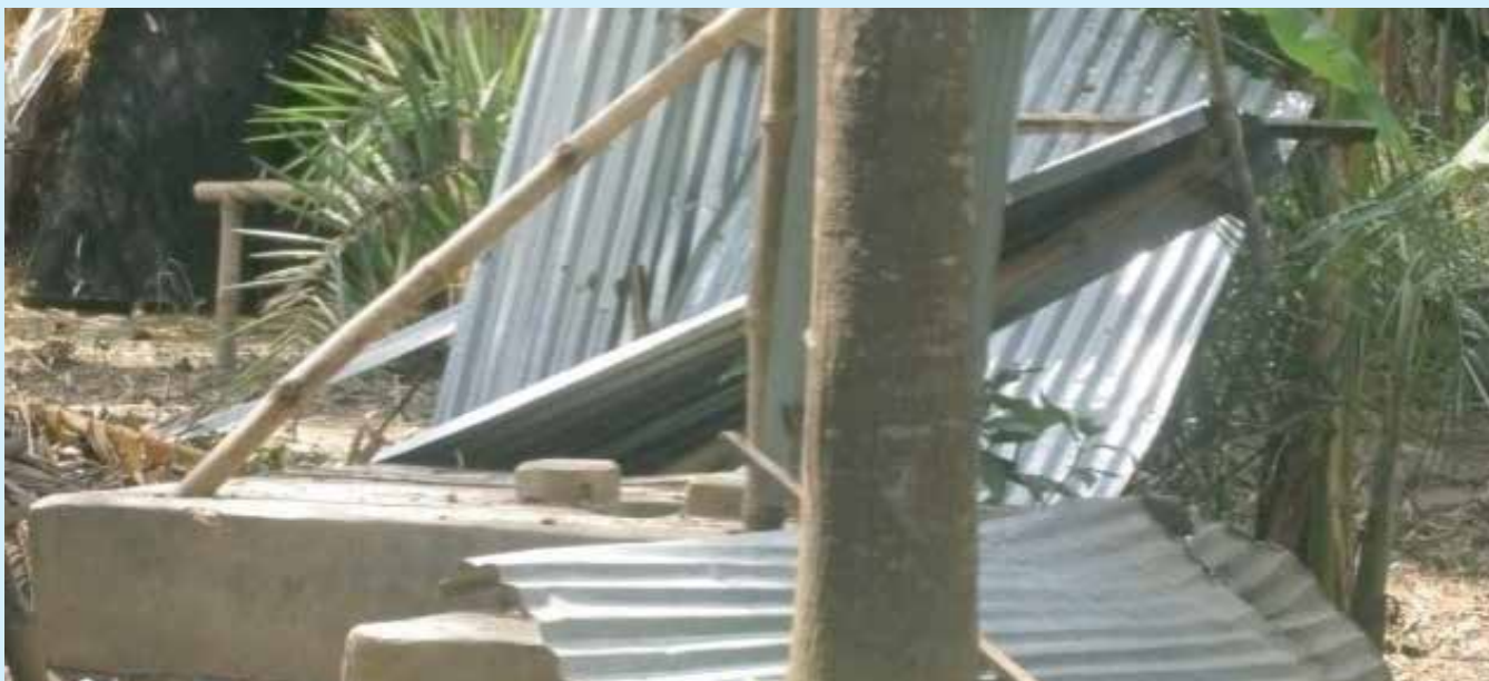
Photograph 7 : Destruction by a storm
