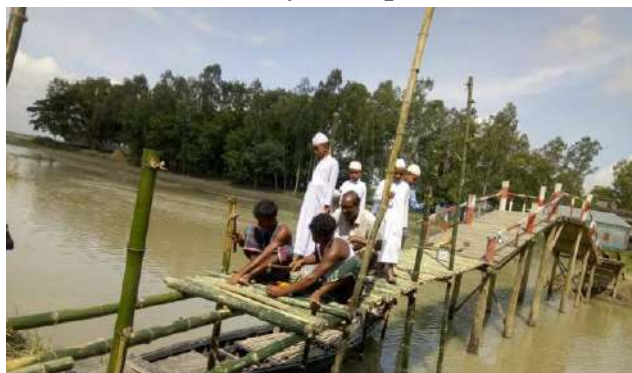
Photo: The bamboo bridge broken in the present flood then repair in a joint venture between VDC & DRR leaders, Dattakandi, Omarpur, Chouhali. Photo Credit: Al- Amin FT ED Date: 26/06/2022
